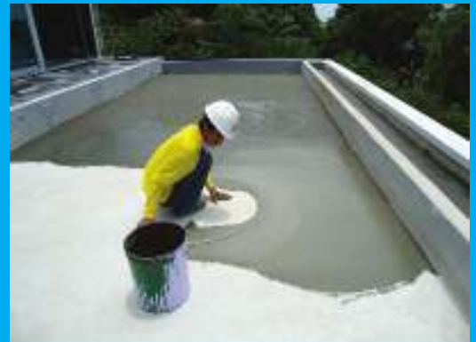
Roof deck water pond waterproofing
